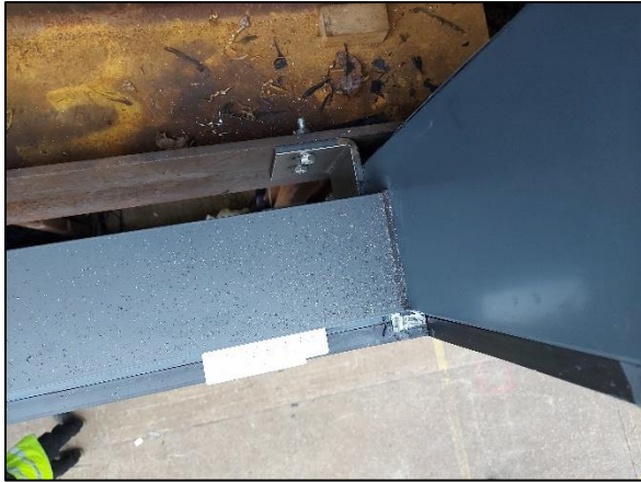
Photograph No. 9 - T connection with glazing removed showing glazing packers
