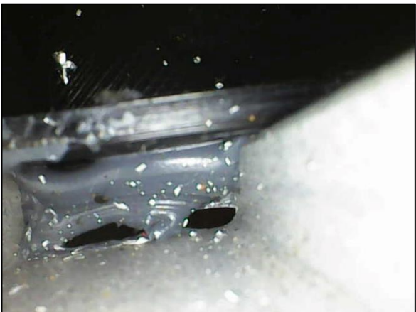
Photograph No. 19 - Sealant inside bottom of mullion
