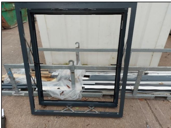
Photograph No. 11 - Opening vent removed
